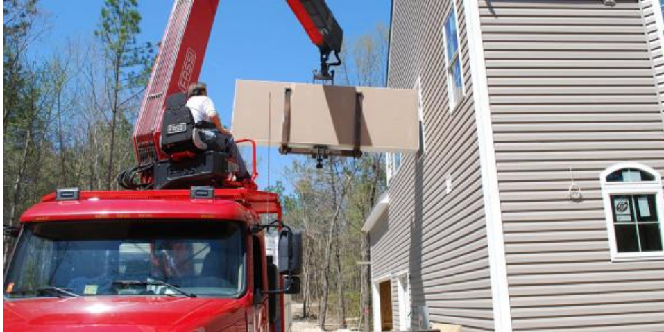
Figure 2. Delivery of drywall to jobsite. Adapted from “FASS Crane Lifting Drywall,” by The Blue Book Network, n.d. Copyright 2015 by Contractors Register.
