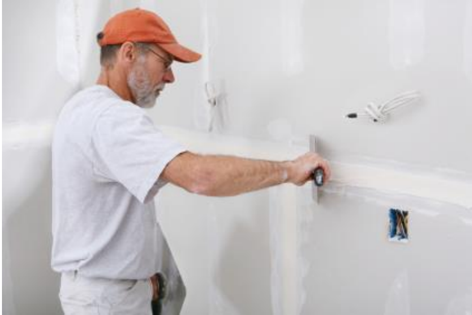
Figure 6. Worker applying joint compound. Adapted from “Craftsman Finishing Drywall Joint,” by Earley Construction, 2009. Copyright 2009 by Earley Construction.
