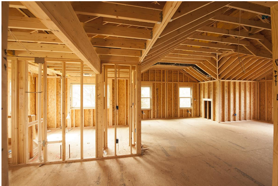
Figure 1. Framing of a house ready for drywall installation. Adapted from “CotY 2013 Award: Entire House, Framed House Structure,” by EDW Builders, 2013. Copyright 2013 by Bob Graham, Jr. Photography.
