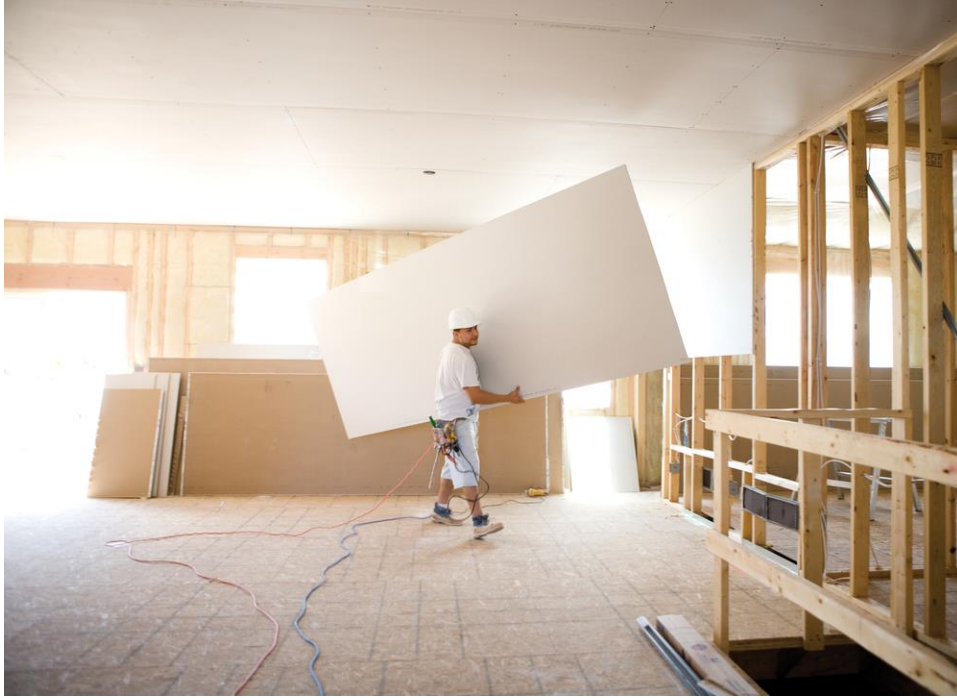
Figure 4. Worker fitting and installing drywall in residential building. Adapted from “Ultralight Sheetrock Drywall Panels from USG,” by Charles and Hudson, n.d. Copyright 2015. by Charles and Hudson.
