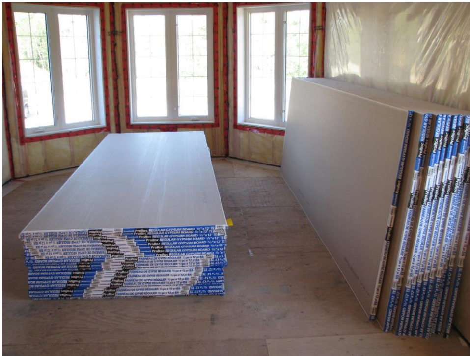
Figure 3. Drywall stacking in building. Adapted from “Nohasslecastle.com,” by Joe, 2011. Copyright 2011 by Joe.
